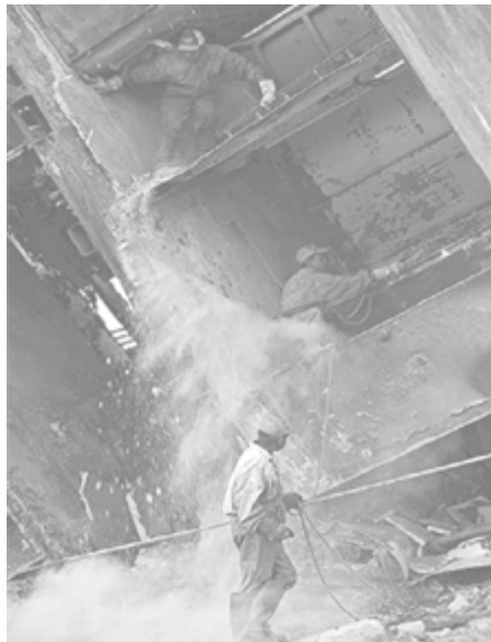
Figure: The hatches and pockets of vessel may contain explosive or inflammable gases, Source: Ship Breaking Activities and its Impact on the Coastal Zone of Chittagong, Bangladesh: Towards Sustainable Management , Young Power in Social Action (YPSA), July 2006
