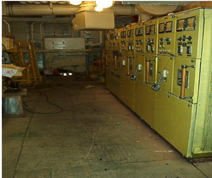
Rubber carpet missing in mail el. switchboard
