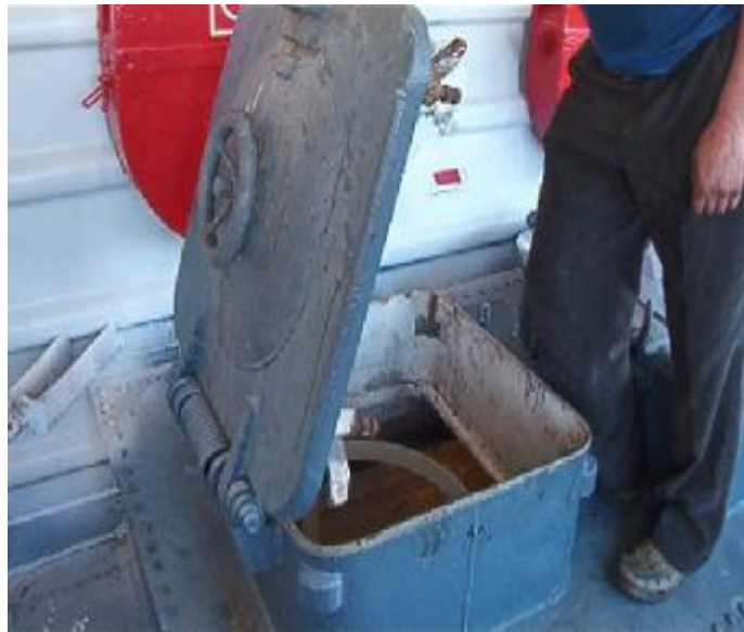
Cover spring broken of the emergency escape engine room
