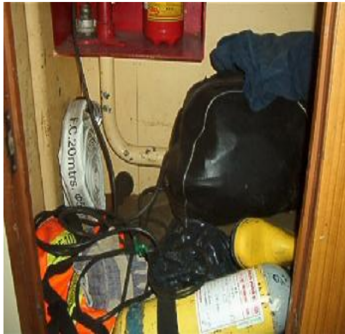
Safety locker – fire equipment mixed
