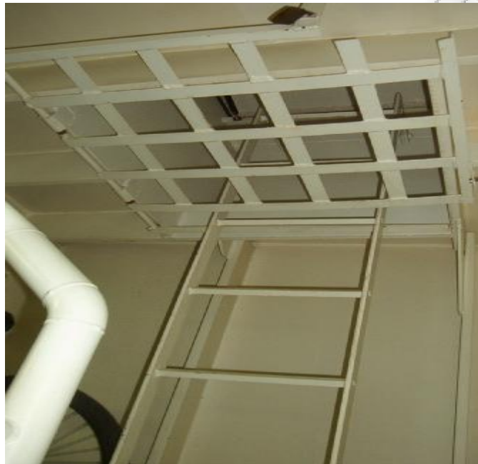
Emergency exit blocked with padlock
