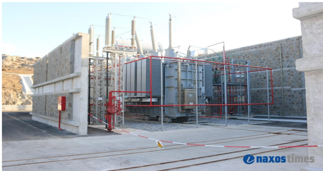
Figure 40: An onshore substation in the interconnected island of Naxos, built with stone, to be in harmony with the local environment. This would be similar with the second described, in this thesis, onshore substation in Karpathos.
