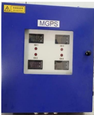
Image. MGPS control panel
