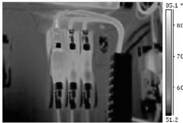
Figure 44. Infrared imaging of a fuse box [1,2]
