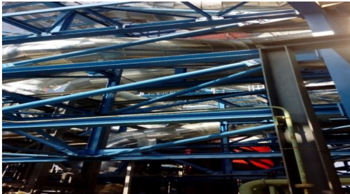
Photo 2.9: Arrangement of the catalyst with a resistance structure at the ICE 1 substation [1]
