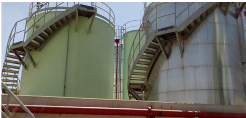
Photo 2.2: Fuel oil storage tanks [1-14].
