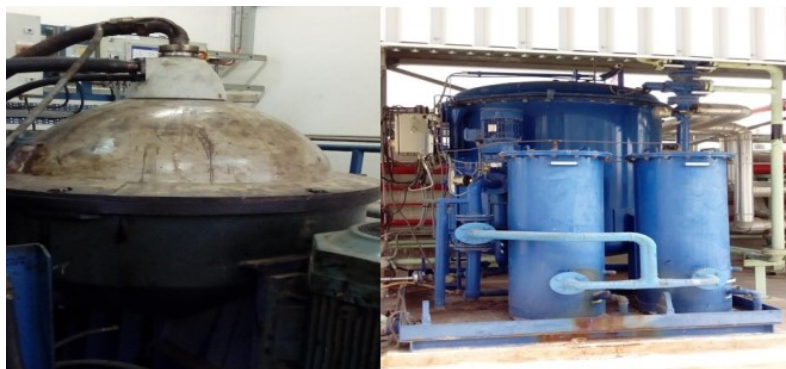
Photo 2.8: a. Fuel oil and b. Water separators [1]
