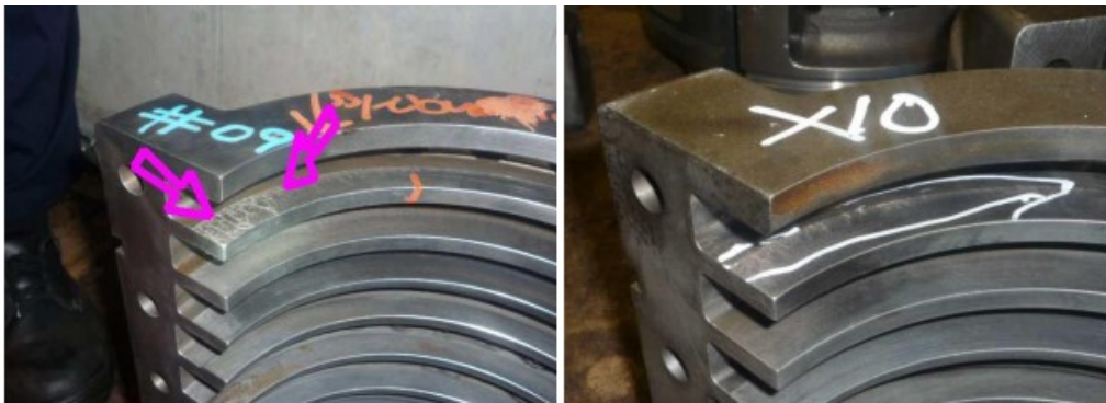
Photo 3.7: Wear in ring grooves due to waste material for ID 9 and 10 Scavenging air receiver [1]
