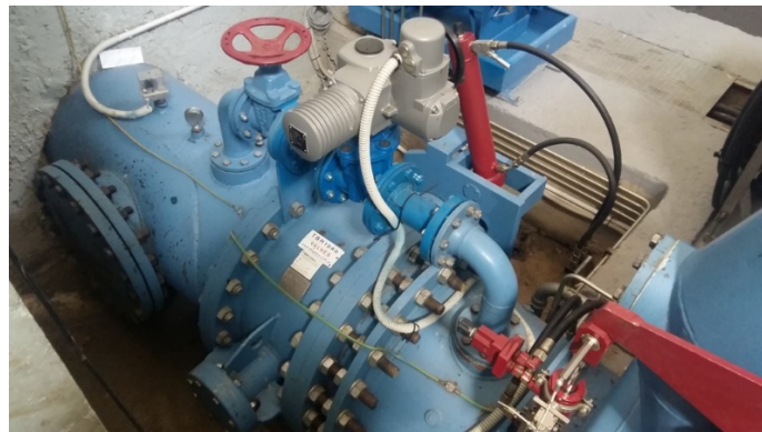
Main Inlet Valve and bypass pipe
