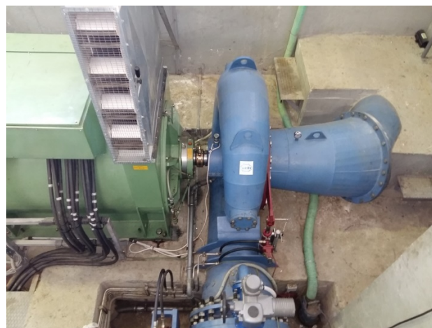
Francis horizontal axis type turbine
