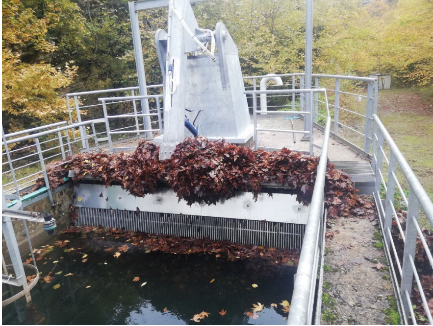
Automatic trash rack cleaner
