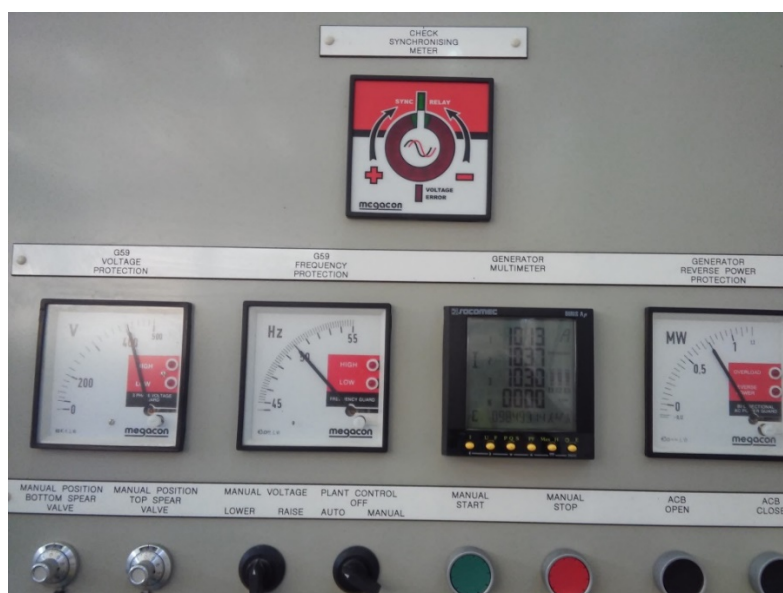
Operation measuring instruments
