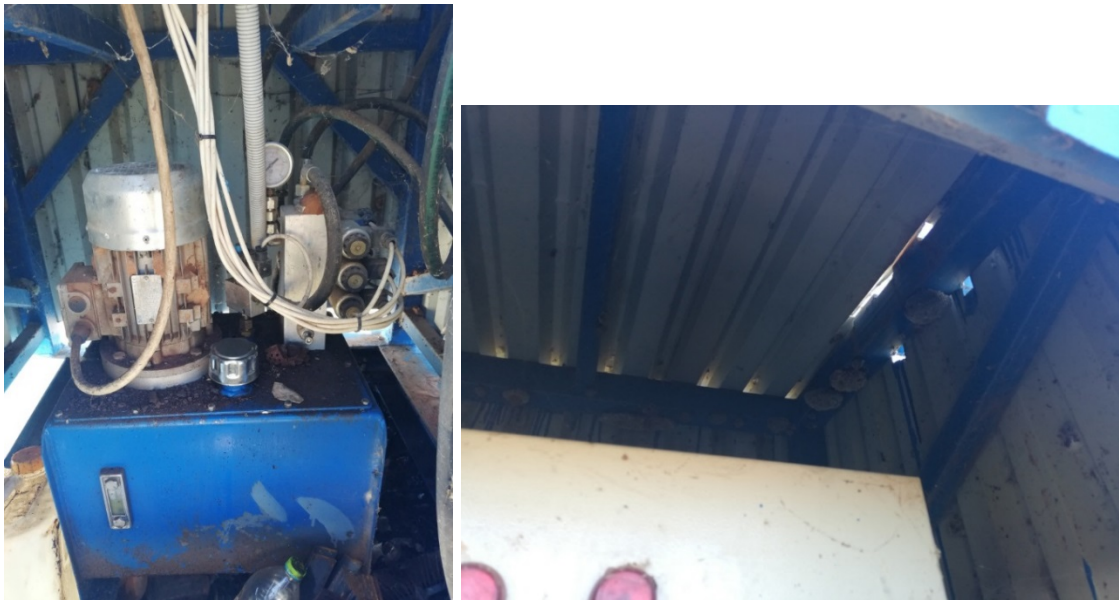
Hydraulic unit and automatic trash racks cleaner control lodge
