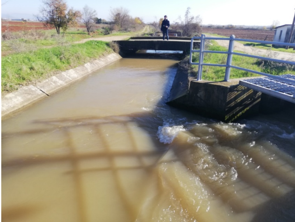
Channel water gate next to the loading tank
