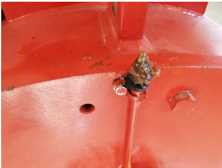
Non Drive End bearing greaser
