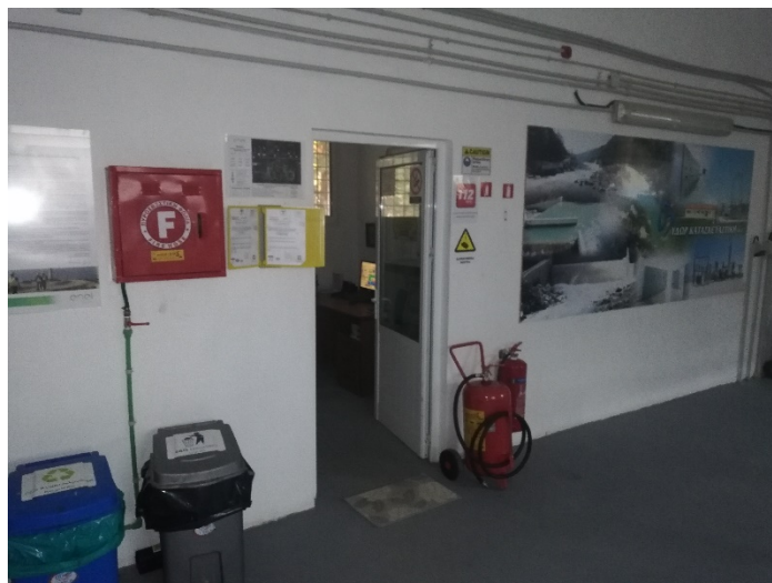
Retread Fire Extinguisher and Fire Nest
