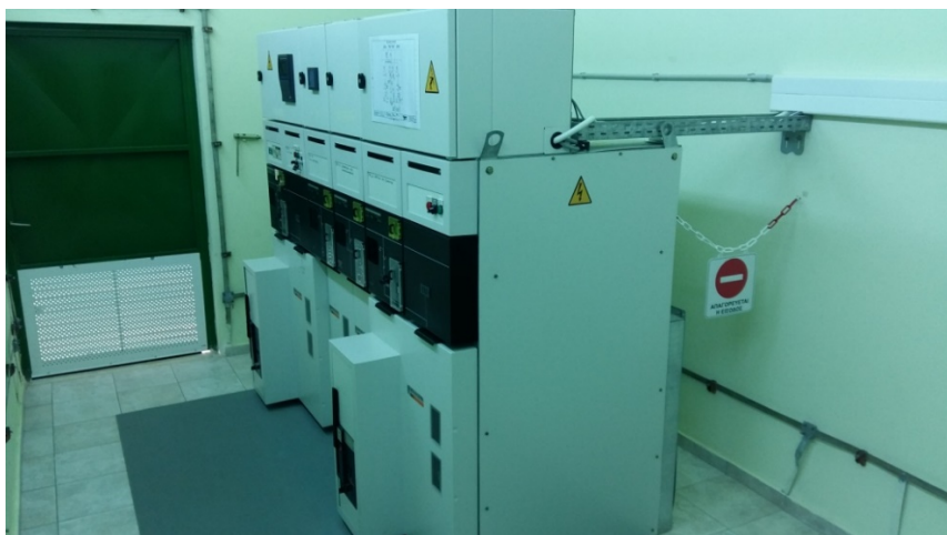
Medium Voltage Cubicles
