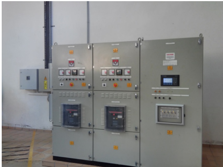
Low Voltage Panel (PLC)
