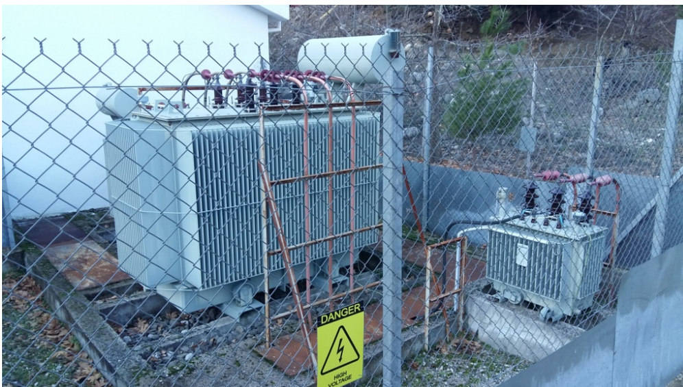
Main and Auxiliary transformers
