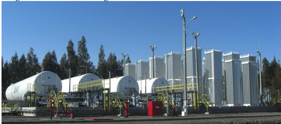
Image 4: Small Scale LNG Regasification Plant
