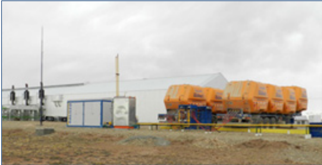
Image 10: CNG Containers at Customer's Site
