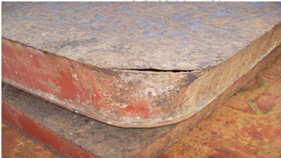
Εικόνες Γ12 & Γ13: Hatch cover pontoons are corroded and cracked
