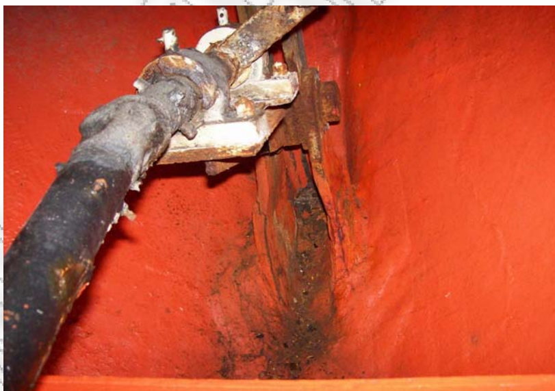
Εικόνα Γ2: Corroded and cracked boat hook supports need to be repaired
