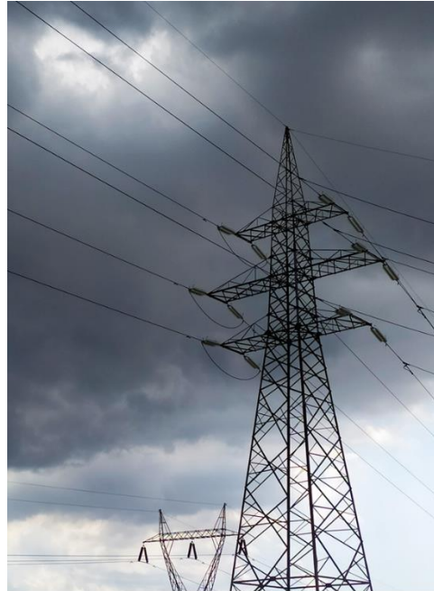
Figure 2.5 Electricity transmission tower
