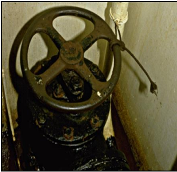
Sea and overboard discharge valves, not in use, are closed and visibly secured.
