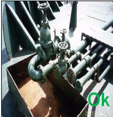
Scuppers and 'save-alls' are effectively plugged and drip trays are in position and empty
