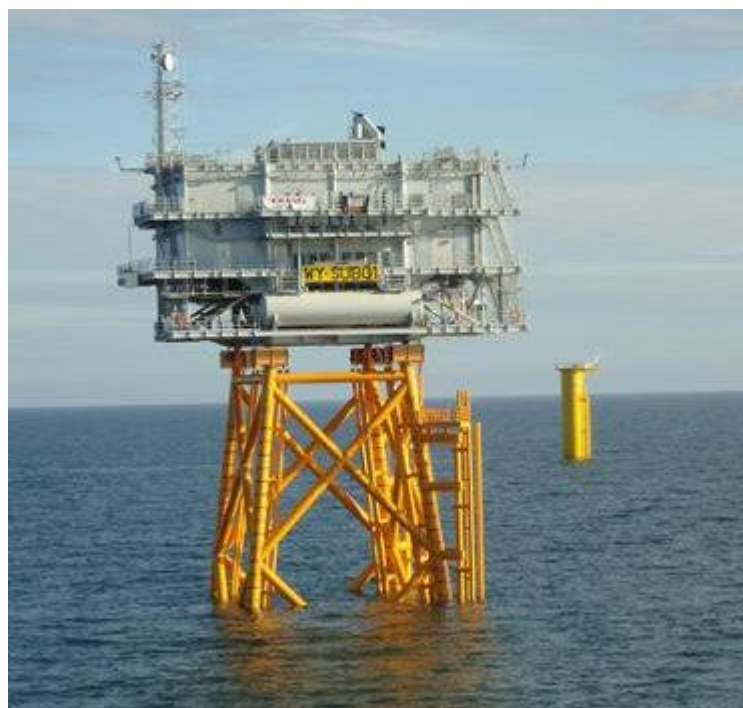
Figure 13: The Offshore Substation (4C Offshore)
