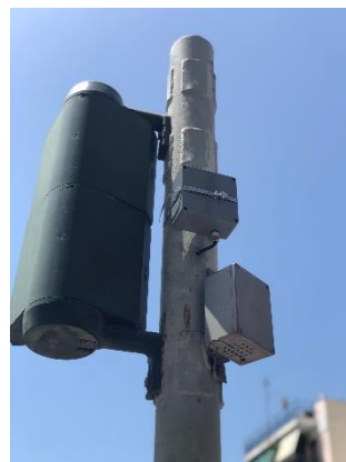
Figure 12.8. Specially mounted external device on a real traffic light located at the junction of Doiranis and Athinas in Kallithea.
