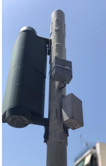
Figure 8.3 Traffic sensor (the field sensor is the upper box).
