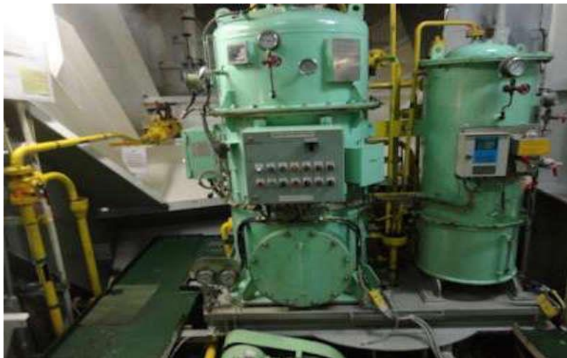
Figure 8: Oily Water Separator
